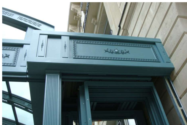
Decorative elements in bas-relief in Acrystal Prima - Exterior glass roofs - Parisian palace - Place Vendôme - Realization Wery Stenger - Paris
